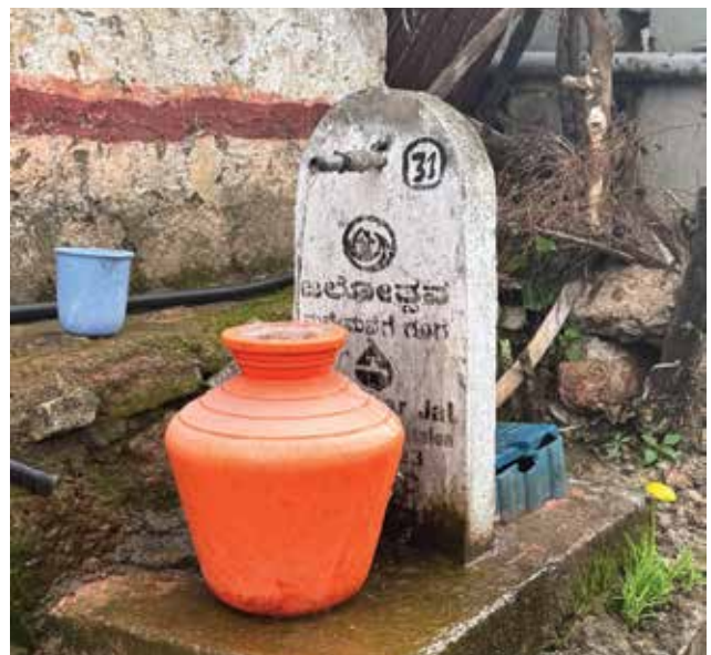
JJM Tap Connection in Bidar, Karnataka
